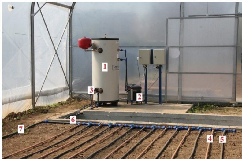
Fig. 1. Irrigation by condensation installation: 1 – water tank; 2 – water chiller; 3 – circulation pump; 4 – copper pipes; 5 – PEHD pipes; 6 – water inlet pipe; 7 – water return pipe
